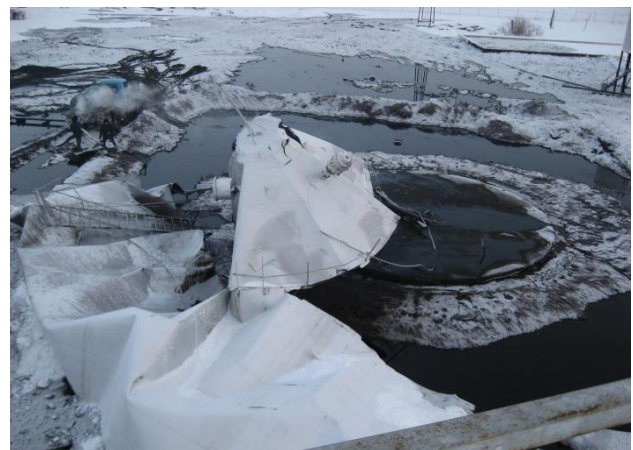
Figure 3. Fracture of the vertical tank RVS-700 №49 with capacity of 700 m 3 .
