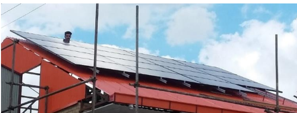
Figure 1. Photovoltaic system in Darian
