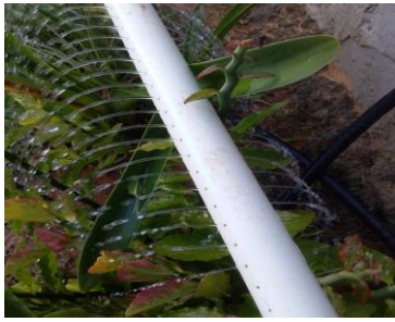
Figure 6. Permeate tube for irrigation
