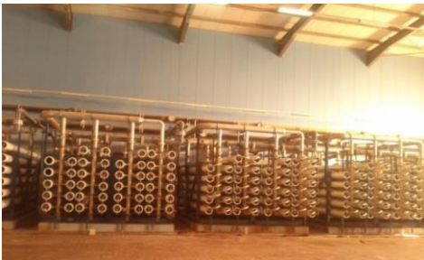
Figure 1. Spiral wound membrane modules in the Tajoura desalination plant
