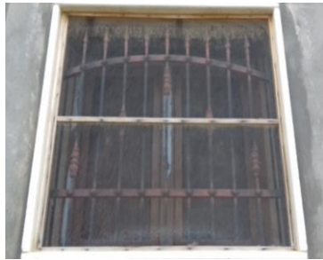
Figure 7. Window's protection from Mosquitoes attack
