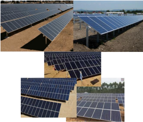
Figure 2. Examples for single line and double lines of PV modules per row
