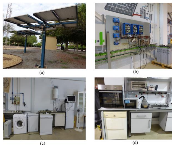
Figure 2. (a) Photovoltaic (PV) generation in the microgrid; (b) Power electronics and batteries; (c) and (d) domestic appliances (loads)
